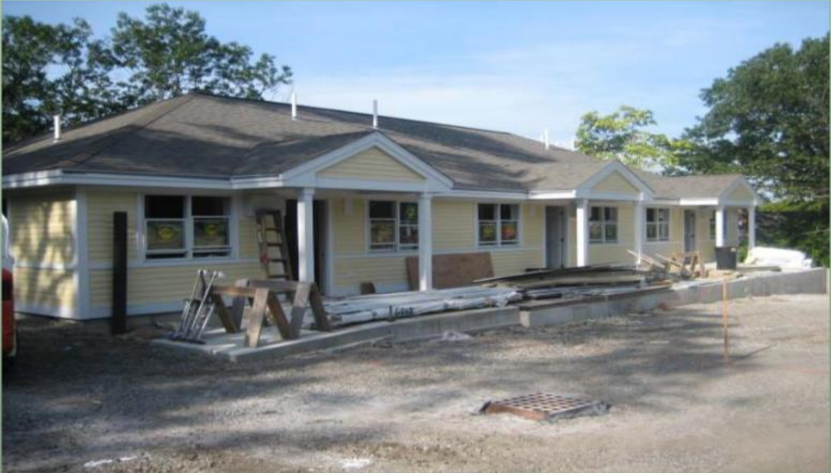
Lynn M. Marcella Residences at James Street (Two Bedroom Homes) CPC provided $75,000 of the $1.3 million project cost
